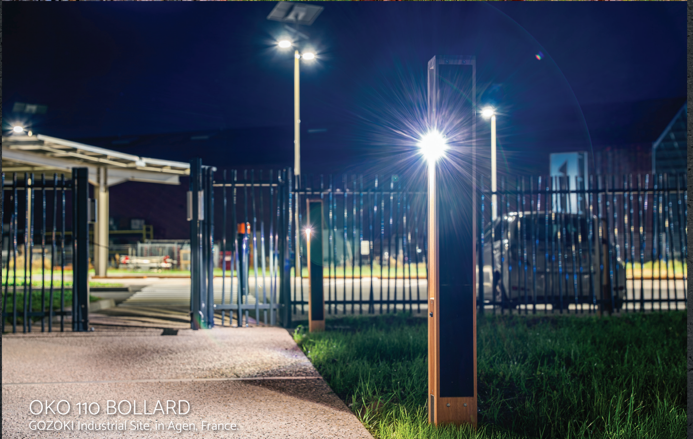
OKO 110 BOLLARD in Saint-Paul Mont Penit, France. Lighting Design : SYDEV
